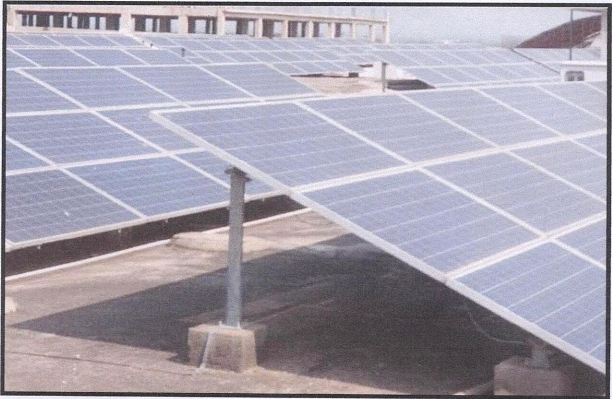
Fig. 2.4- Rooftop solar panels
